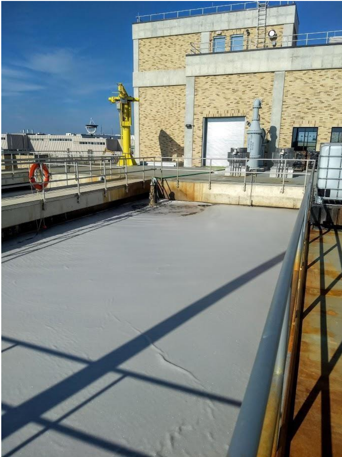
Figure s3: Source of filtrate for pilot MFC system, filtrate reactor feed head tank at Filtrate Treatment Facility, DC Water Blue Plains, Nov 29 2018
