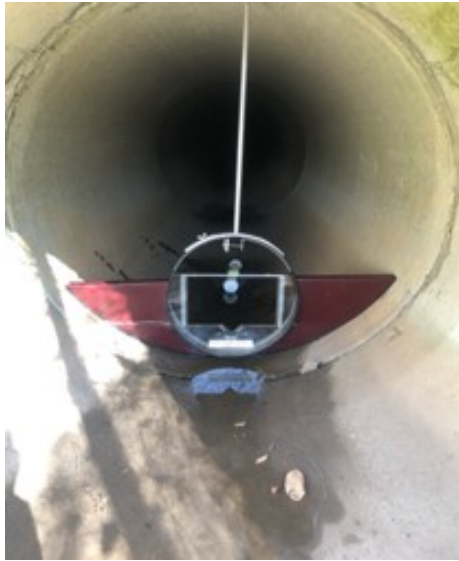
Figure A.4: A Thel-Mar volumetric weir mounted within the outfall pipe of terminal dry detention Pond 6 along with the water level pressure transducer, within a protective PVC housing, mounted six feet into the pipe behind the volumetric weir.
