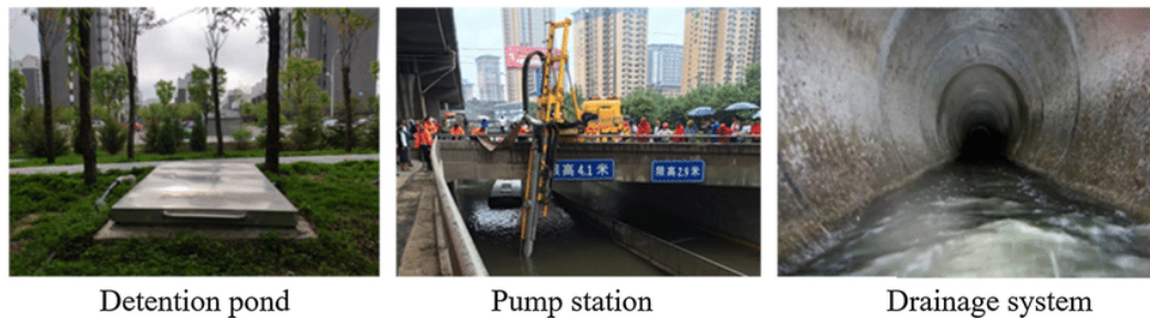
Figure 1.2: Examples of traditional grey infrastructure utilized for stormwater management in cities across the United States. These infrastructural systems were the primary techniques used throughout the “Drained Cities” and “Waterway Cities” paradigms [21].
