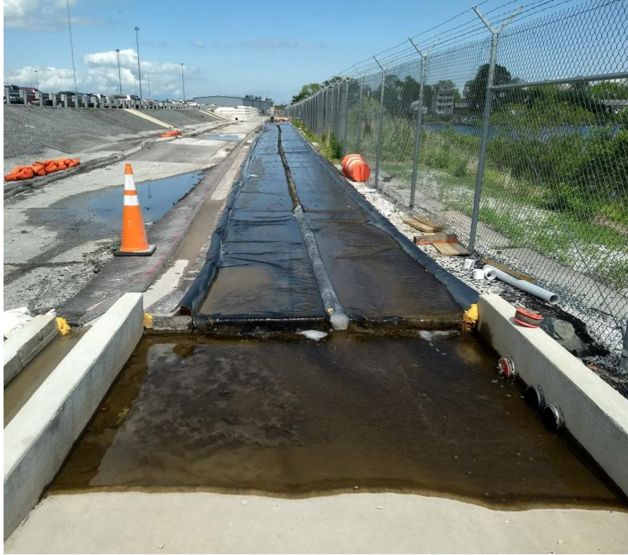
Figure 2.1: Pilot-scale algal turf scrubber (ATS) installed at the Port of Baltimore Dundalk Terminal (Baltimore, MD, USA).
