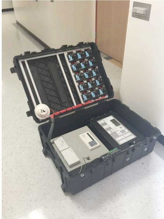
Figure 2.2: Customized Siemens Fire Safety System – Fire Alarm Control Panel A multi-criteria fire detector, Model FDOOTC441, was determined to be an optimal sensor as it can measure multiple types of data using optical, thermal and CO sensors. Smoke detectors are a prevalent reliable sensor used throughout most buildings, as they are required in the United States by most state and local laws as defined by NFPA 72 (National Fire Protection Association, National Fire Alarm and Signaling Code). Direct measurements of temperature and smoke obscuration as well as temperature, smoke, and CO alarms were relayed to the panel. The multi-criteria smoke detectors were located throughout the MFRI structural fire fighting building. The coordinates of the smoke detectors are shown in the Appendix. The origin is taken from the bottom left corner of the BIM as shown in Figure 2.3. Each floor
