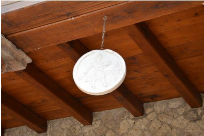
Figure 37. Looking up at T44, Side A, 2015, House of the Telephus Relief, Herculaneum. (Photo by Mentnafunangann, CC BY-SA 4.0).
