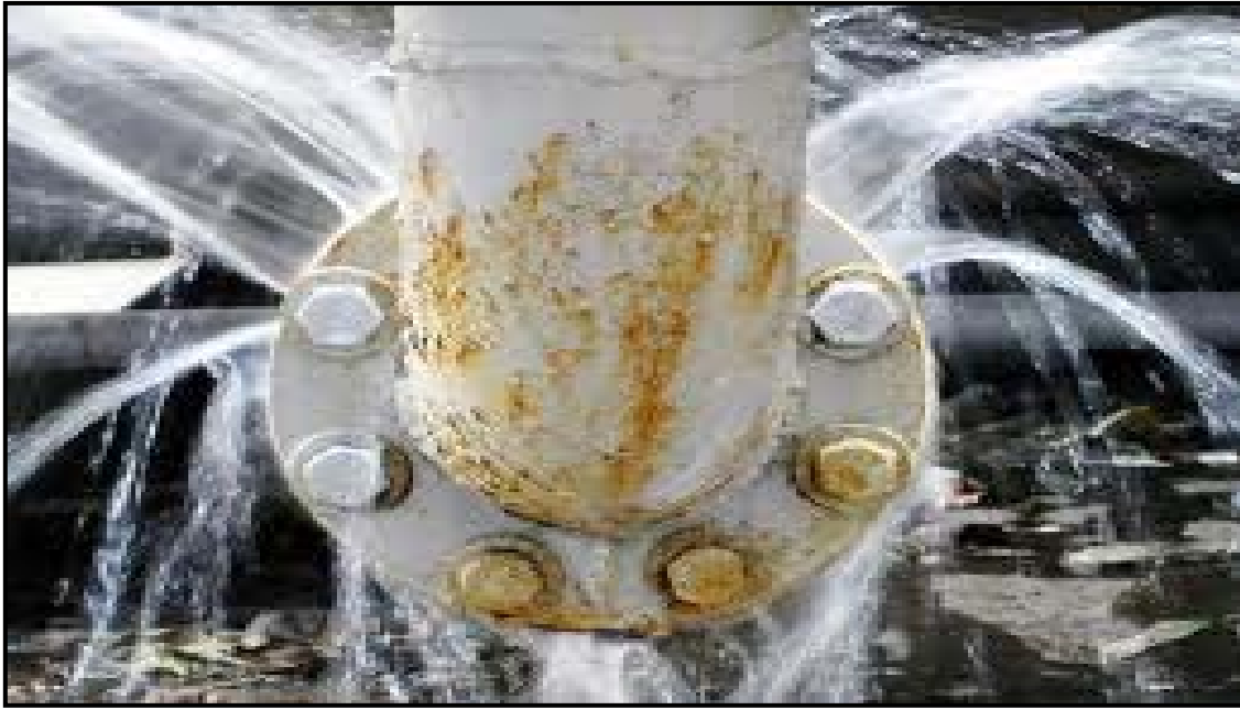
Figure 1-3. Water Leakage in a Joint
