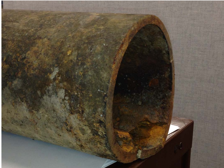
Figure 3-5. Pipe Graphitization Corrosion
