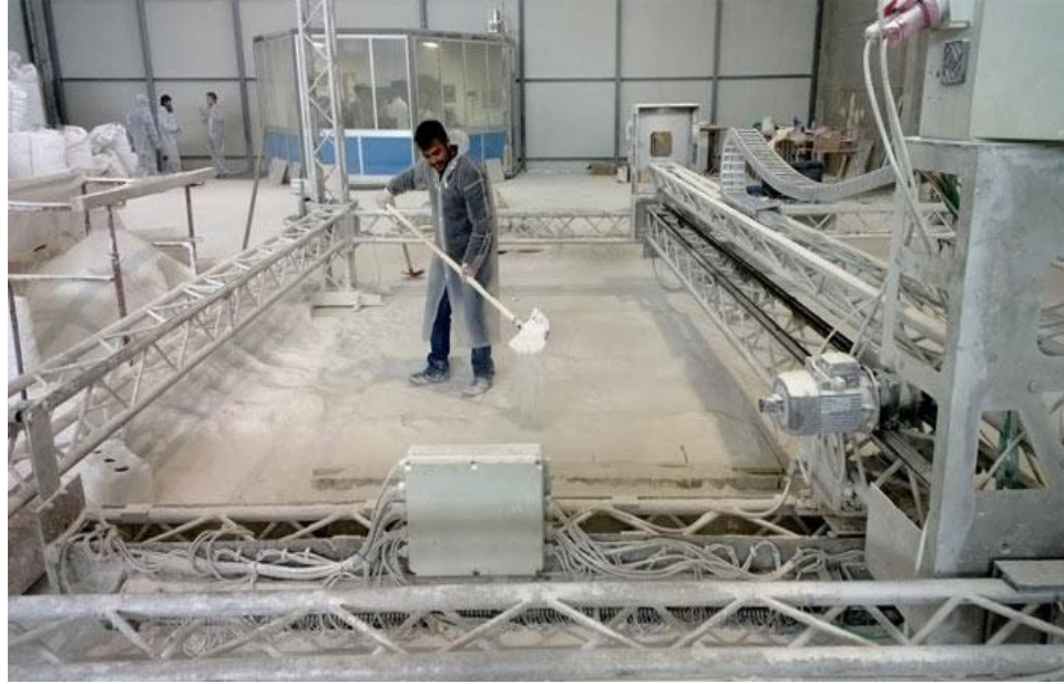
Figure 7. D-shape's printer (Jamie, D., "3D printing: The Future of Construction", January 31 st 2018).
