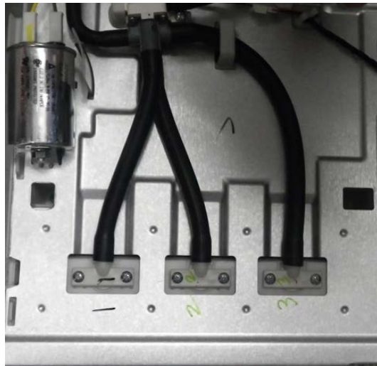
Figure 14: Pipes collecting condensed water
