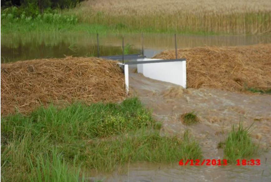
Figure 2-2. Tracom Cutthroat Flume Installed at the Influent End of the System
